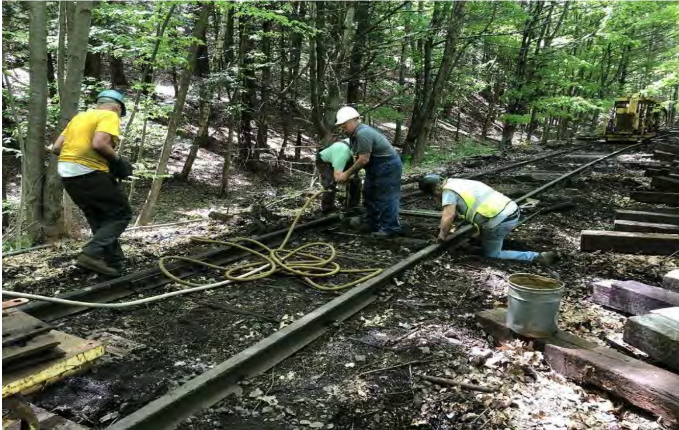
CMRR crews hard at work replacing ties near MP 8 in Stony Hollow in 2019.
